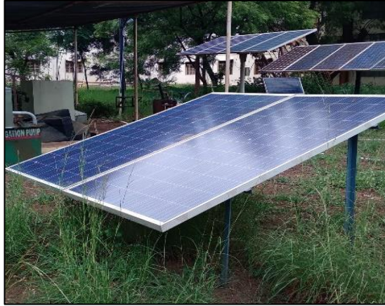
Figure 4: Solar PV Panels Used for The Pumping
